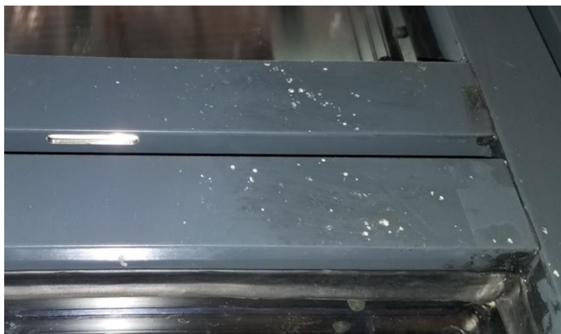
Drain slot out from the glazing stop
